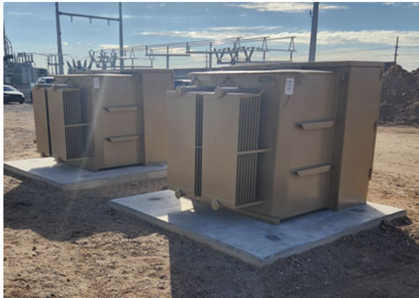
Figure 10 Typical Auxiliary Power Transformer
